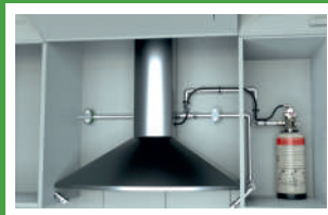
Residential Kitchen Suppression Systems
